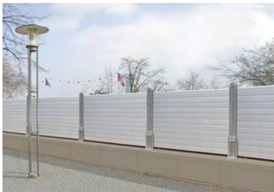
Photo 4: Low foundation wall with demountable flood wall.
