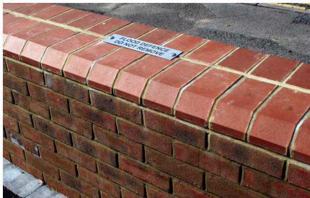
Photo 9: Example of permanent flood wall installation.
